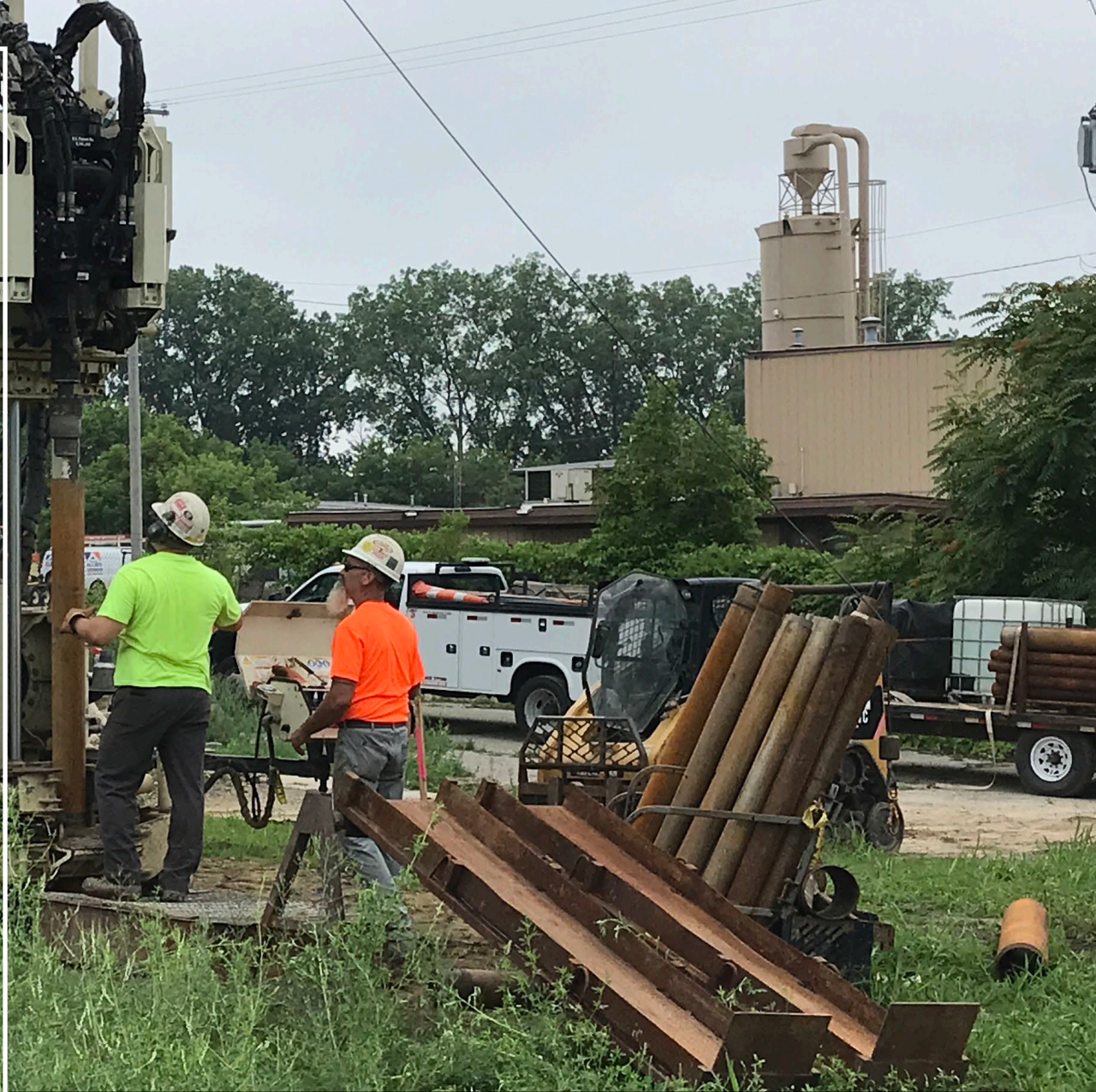
Picture: Workers at Spartan Chemical Company Superfund site where contaminated soil will be excavated in 2022
